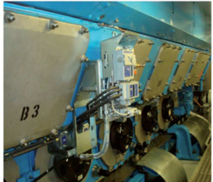
Main engines after conversion to SCHALLER AUTOMATION OMD VN215/87 plus
