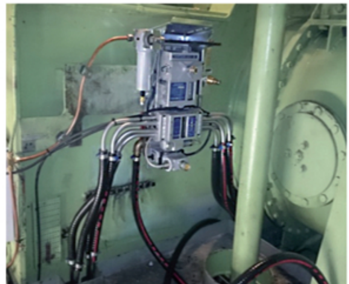
Main engines after conversion to SCHALLER AUTOMATION OMD VN215/87 plus
