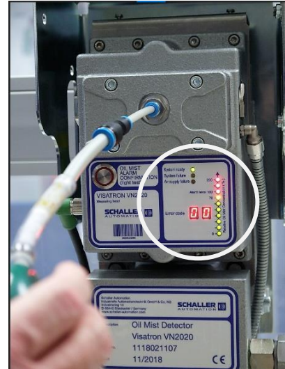
Figure 77: Wait for the Alarm LED to come on
