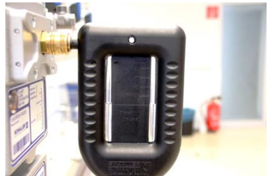
Figure 149: U-tube manometer on inspection cover
