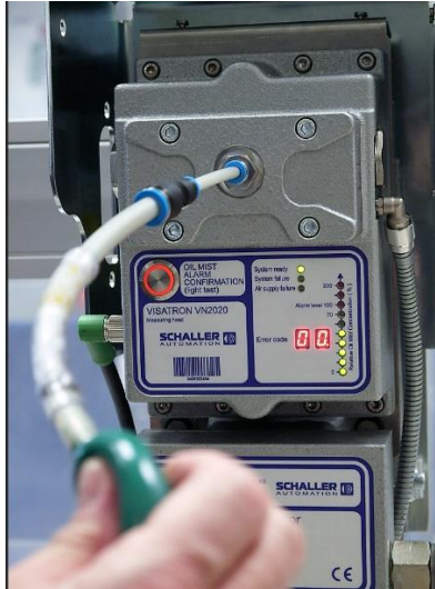
Figure 76: Pump smoke into the measuring head
